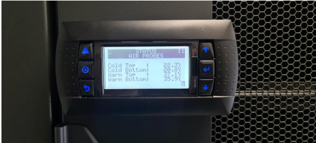
Figure 53: RackChiller Rear Door Display
