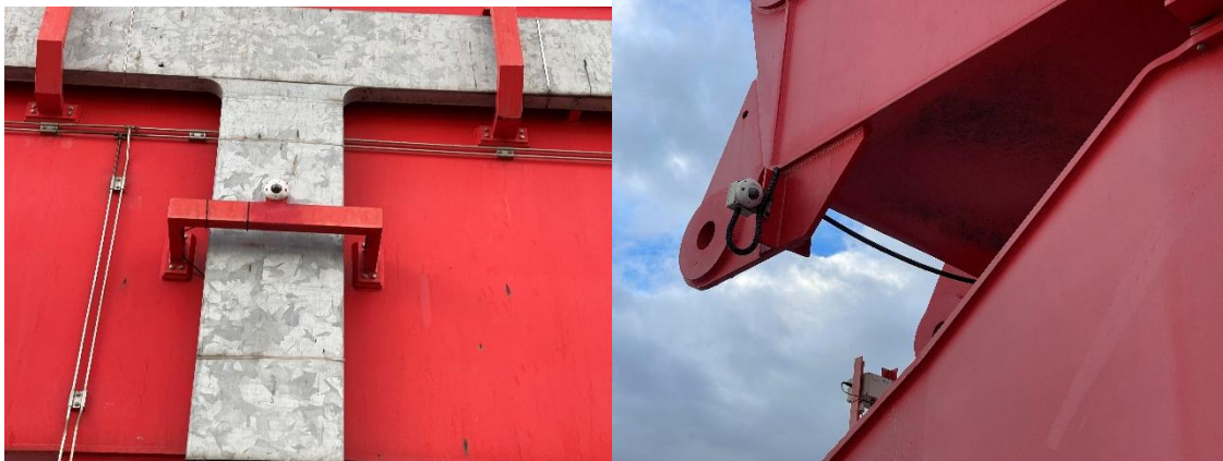
Figure 182. Pilot 4 IP Cameras installed at the STS crane gantry legs
