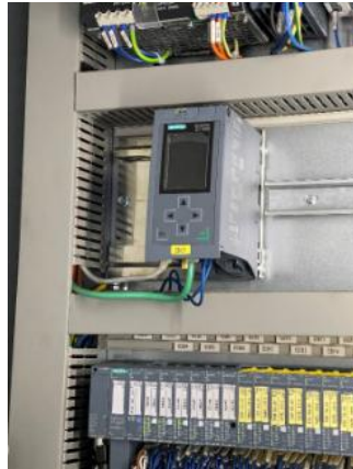
Figure 161. STL Crane PLC
