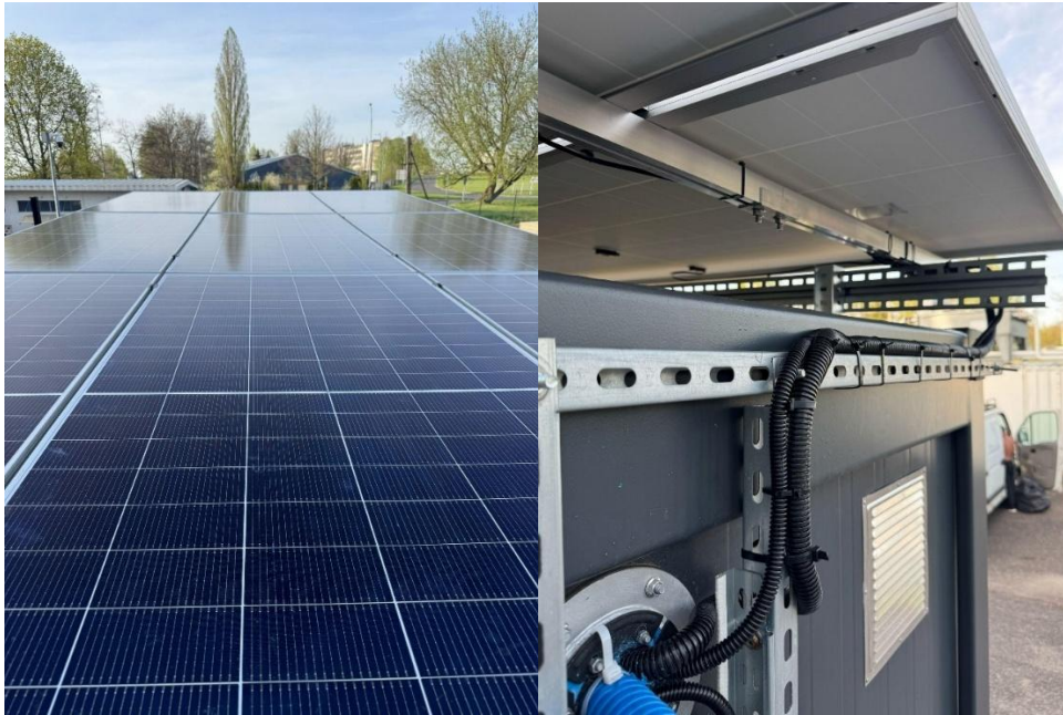
Figure 130. Pilot 2 Container connection to PV
