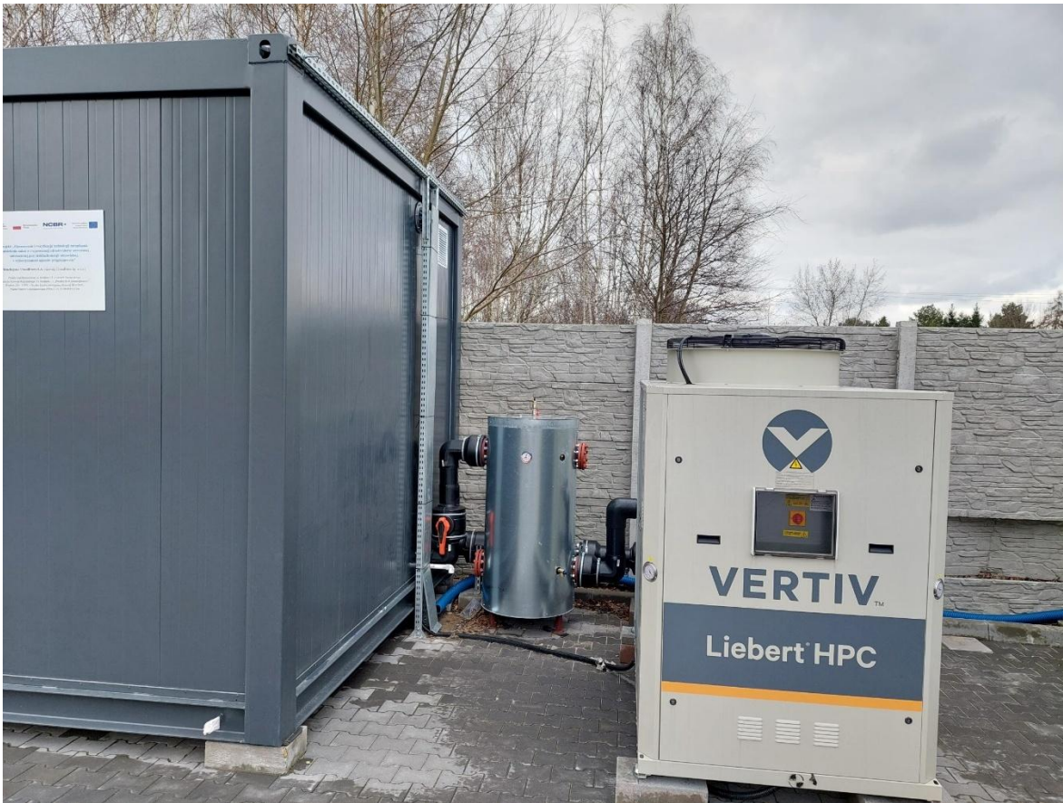
Figure 106. Cooling system installed near the CF container
